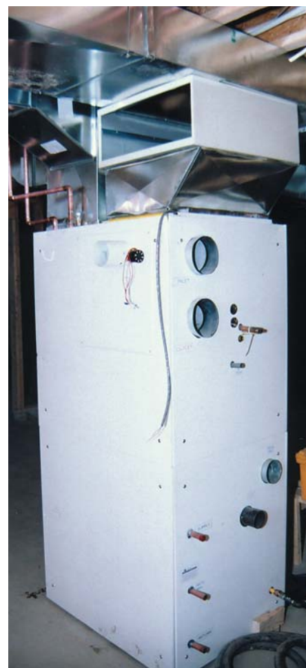
Hookups on the integrated heating unit, incomplete at the time of P&HVAC's visit, are straightforward.
