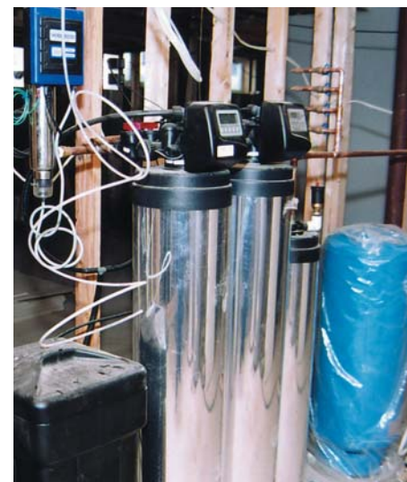
The rural well system operates through state-of-the-art water treatment equipment.
